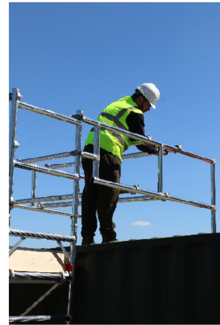
Move your 2 guardrail braces from the unit further out on the roof guardrail
