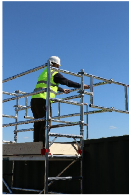
Add 2 additional braces to the roof guardrails from behind your existing guardrail
