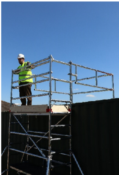
Move the 2 braces again to the end of the roof guardrails from behind your existing guardrail. Then put the temporary guard braces to the back of the unit.
