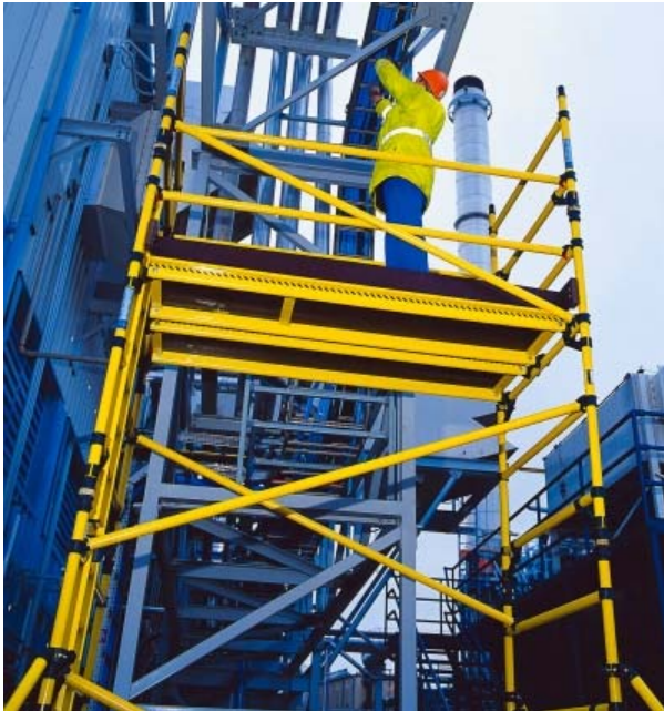
Zone 1 Industrial GRP Towers
